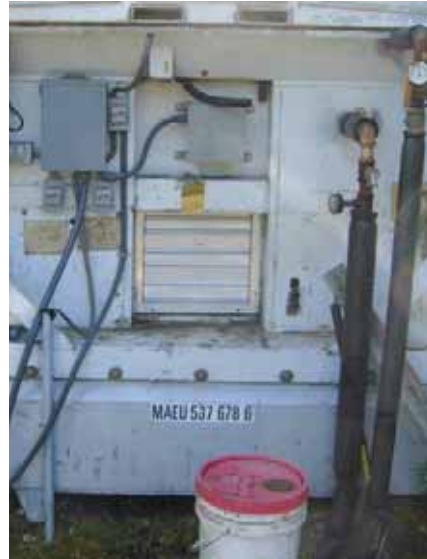
Kiln controls are located on the rear wall of the container.
