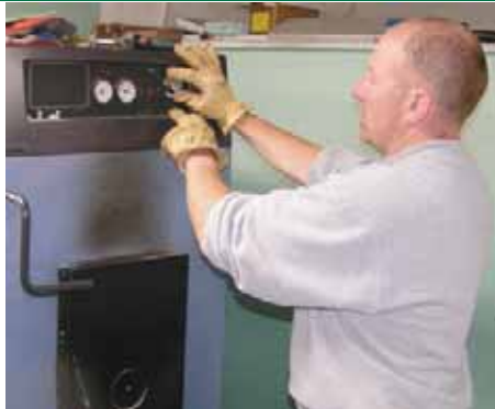
Travis adjusts the temperature shut-off control. The dial indicators to the left are boiler pressure and boiler temperature.
