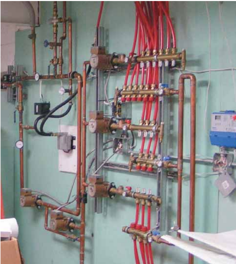
Travis Creswell's storage and distribution system. Note the number of gauges, pumps, and valves. Travis is meticulous in monitoring his furnace.
