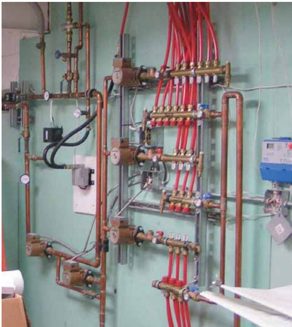
Travis Creswell's storage and distribution system. Note the number of gauges, pumps, and valves. Travis is meticulous in monitoring his furnace.
