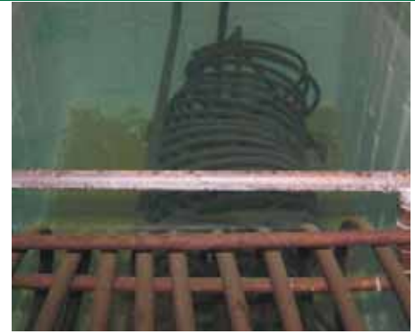
Inside the heat storage tank, showing the heat exchange coils to the boiler (rear) and the domestic water heater (front).
