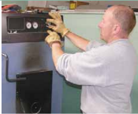
Travis adjusts the temperature shut-off control. The dial indicators to the left are boiler pressure and boiler temperature.
