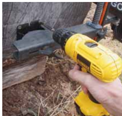
Attaching the bracket to the end of the log. The Big Mill uses a bracket bolted on to each end of the log to hold the guide rail. These must be leveled at both ends so that the chain saw cuts a straight line.
