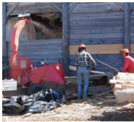
Out behind the wood shed at the VanAlstyne farm, the wood chipper discharges into a chip bin.
